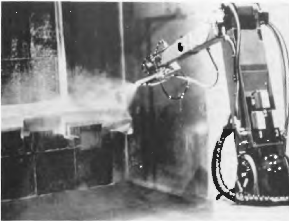
Robot paint machines, like the one shown here, are being used to simplify the painting process and improve control of pollutants.
